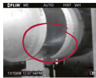
Gas leak in a petrochemical plant
